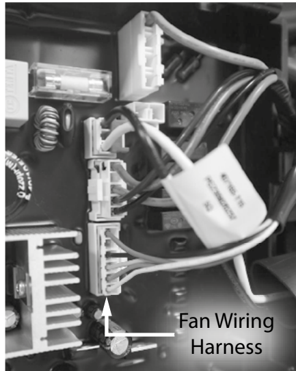
Figure 1 - Locate fan wiring harness on control board
