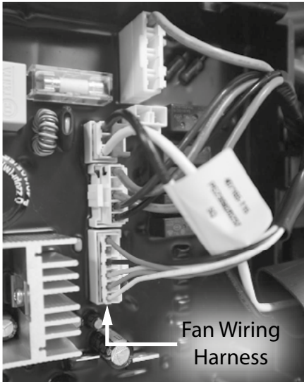
Figure 3 - Locate fan wiring harness on control board
