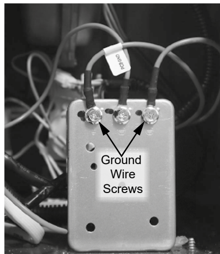
Figure 2 - Location of ground wires
