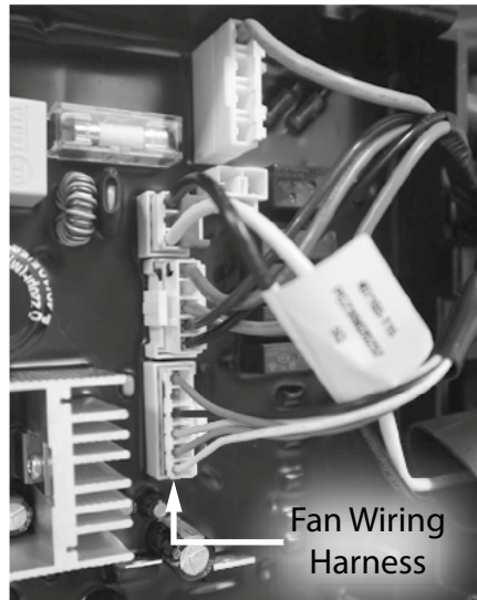
Figure 1 - Locate fan wiring harness on control board
