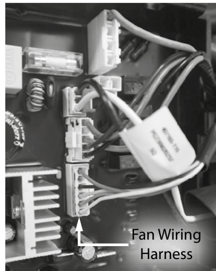
Figure 1 - Locate fan wiring harness on control board
