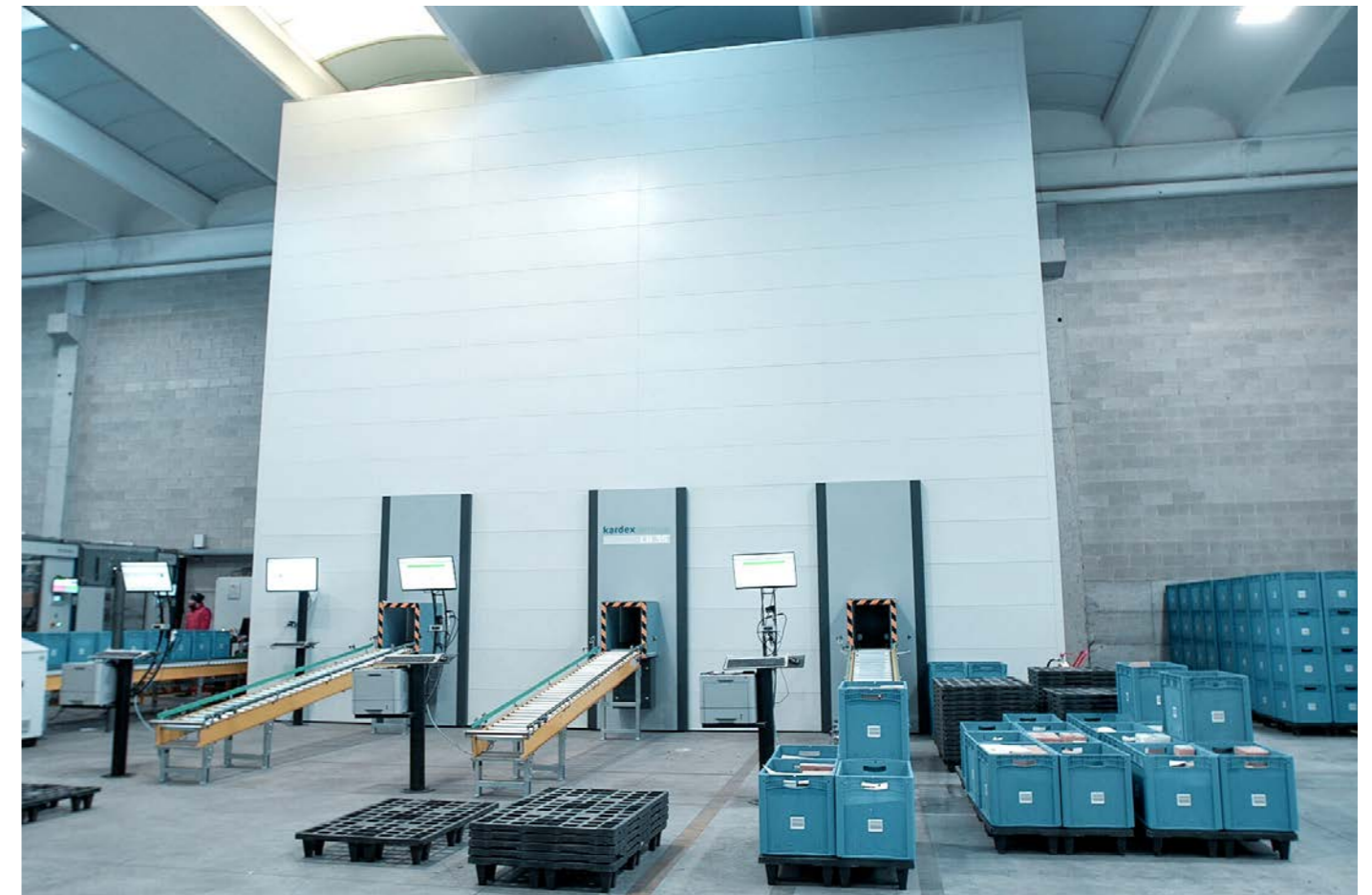
A Kardex Miniload-in-a-Box serves as a simple consolidation buffer with three bin openings.
