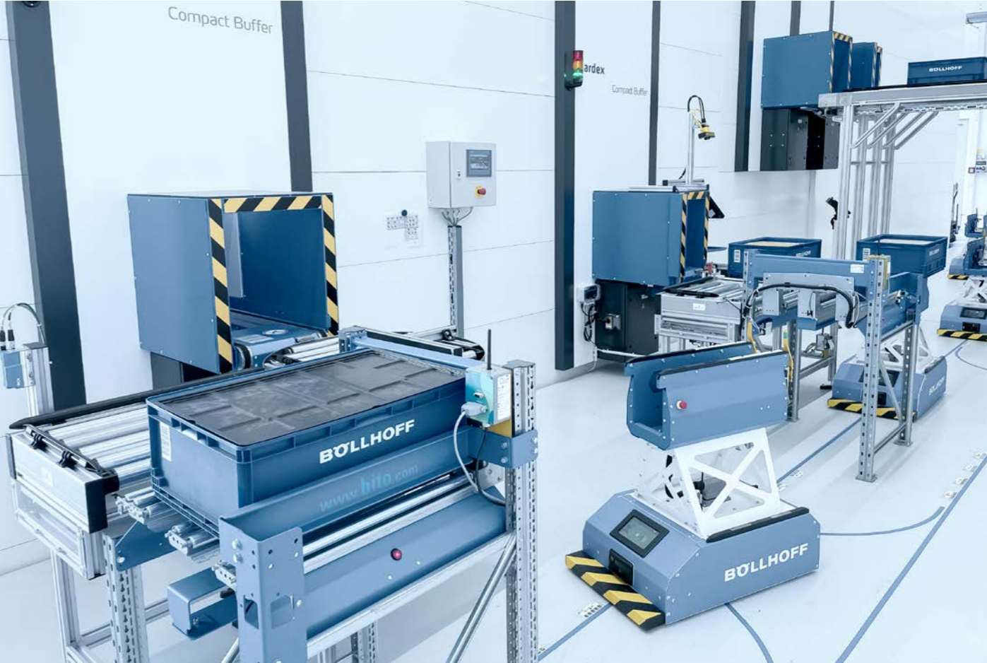
Automated storage and retrieval with AGVs
