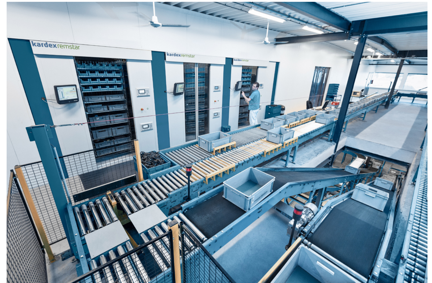
Kardex Horizontal Carousels with conveyor system
