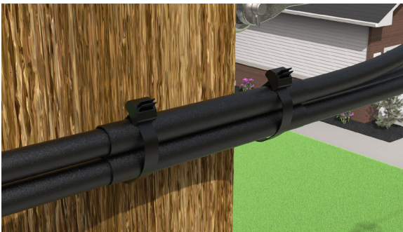
Cable Abrasion Protectors Installed on Cables
