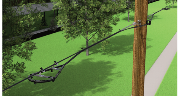
In-Span Storage Installed on ADSS Cable
