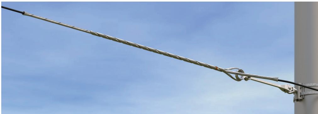
FIBERLIGN Medium Tension Dielectric Dead-End Installed on Steel Pole with Thimble Clevis, Extension Link, and Banding Bracket
