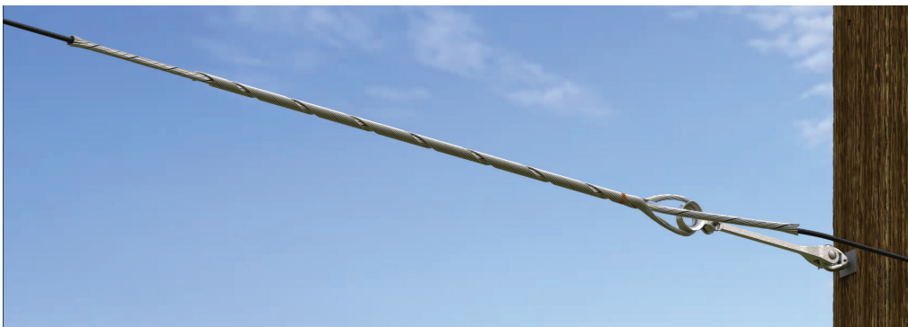
FIBERLIGN Semi-High Tension Dielectric Dead-End Installed on Wood Pole with Thimble Clevis and Extension Link
