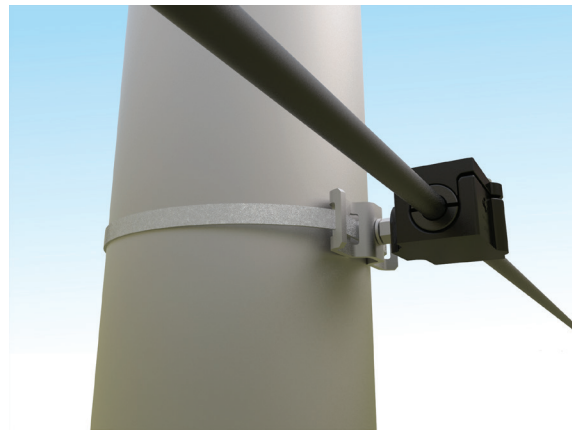
Dielectric Support Banded to Pole
