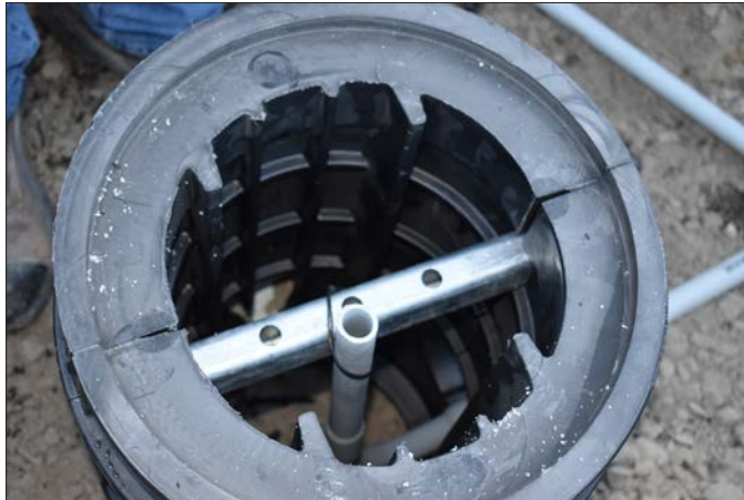
Conduit can be tie wrapped or wire tied to the middle bar for support.
