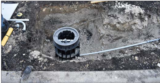
Ground prepared for installation of foundation; conduit ran and routed through open port to middle bar.
