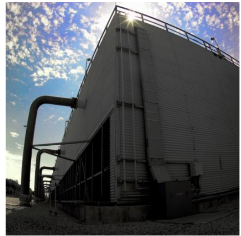
Figure 1: Cooling tower pipes
