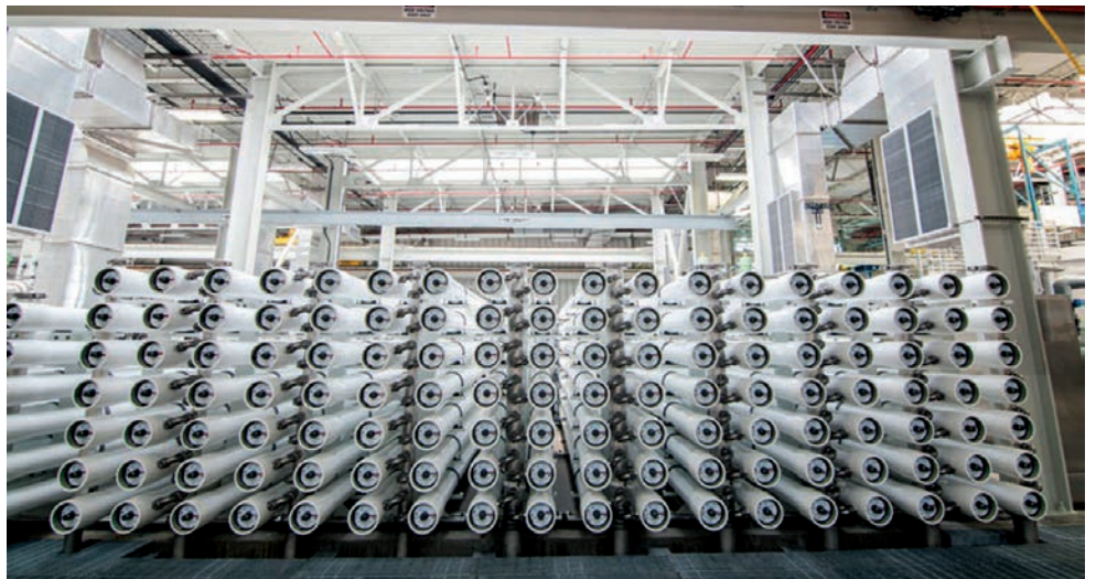
Orange County Water District Potable Water Reuse Facility (Fountain Valley, CA)
