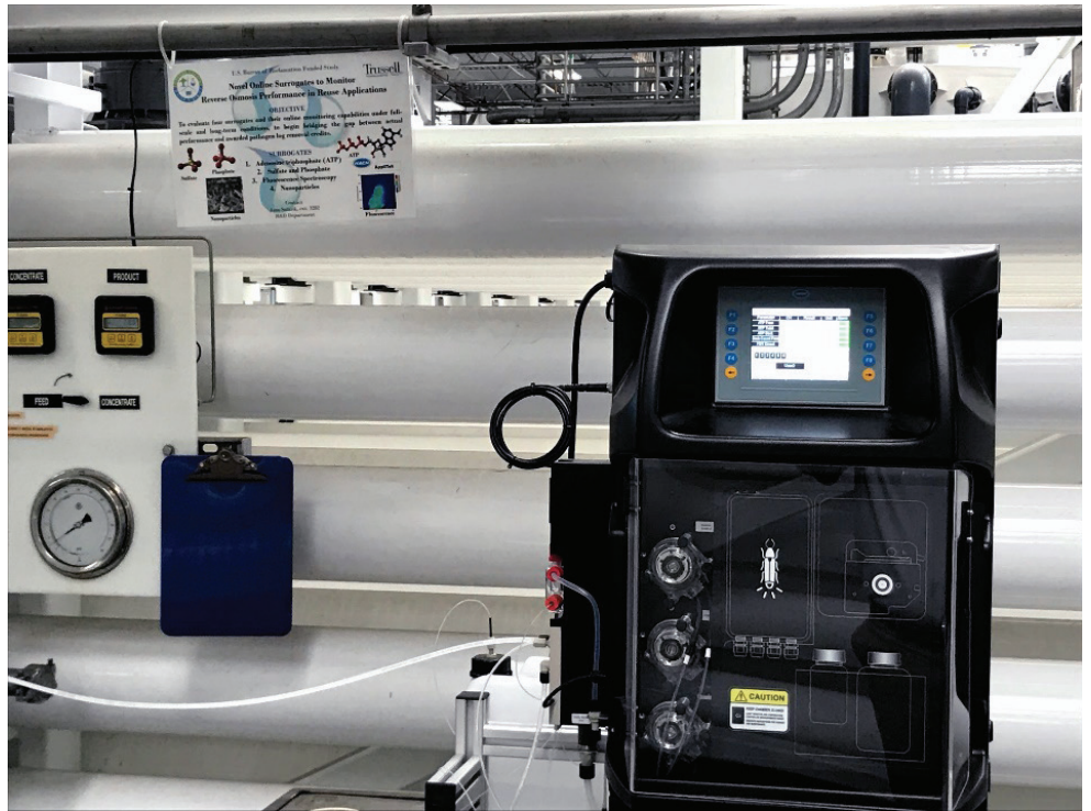
EZ7300 ATP Analyzer installed
