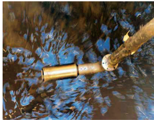
The SOLITAX sc Turbidity and Suspended Solids Sensor attached with fixed-point mount is lowered into the mixed primary sludge feed box feeding the DAFT tanks. Online measurement of solids loading, coupled with flow rate, controls dosing of polymer to the DAFT process.
