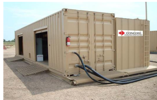
Figure 2: Concord Energy onsite treatment skid
