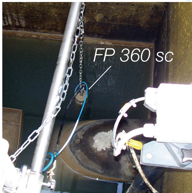
Figure 1. FP 360 sc oil-in-water probe installation in inspection chamber after oil/water separator
