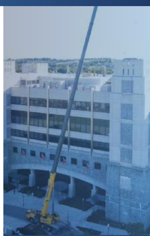
A large crane hoists the colossal MatSing Lens antennas to the apex of Lane Stadium's primary structure for installation by our expert team.
