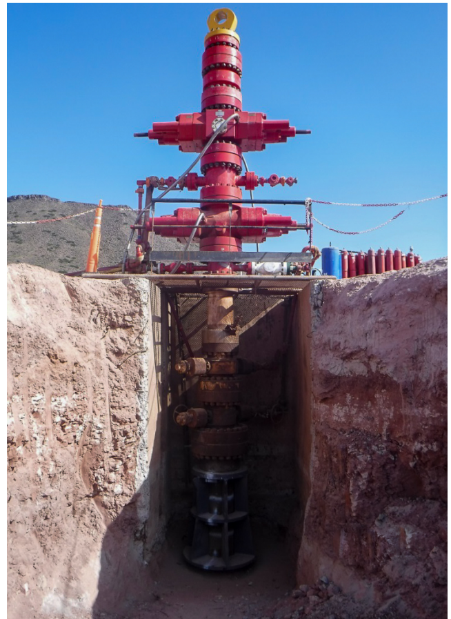
20-in. casing repair: Trench and cellar view with tensioning/capping system and strand jack installed.
