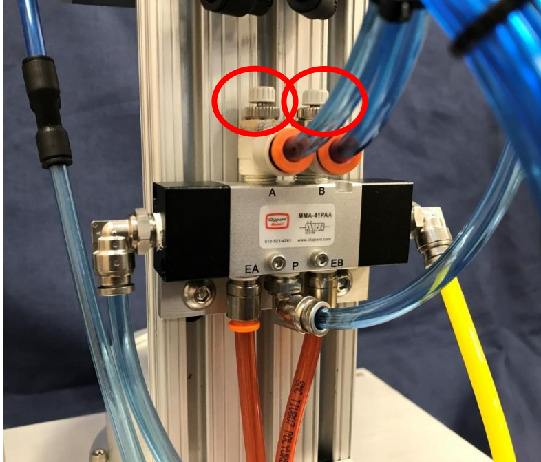
Figure 10. Operating Valve and Flow Controls
