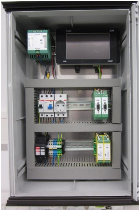
Figure 5: Example of a Standard Lufft UMB Control Cabinet
