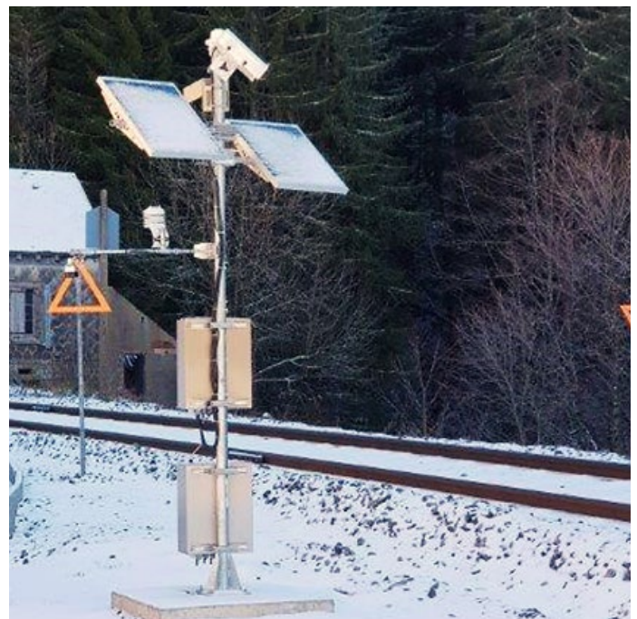
Railroad weather station with a snow height sensor Lufft SHM31 and a compact weather sensor. Credit: OTT HydroMet
