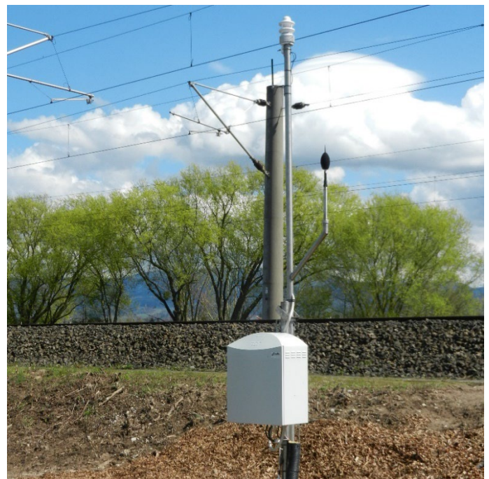
Noise monitoring station at a rail track including a Lufft WS600 weather sensor. Credit: OTT HydroMet
