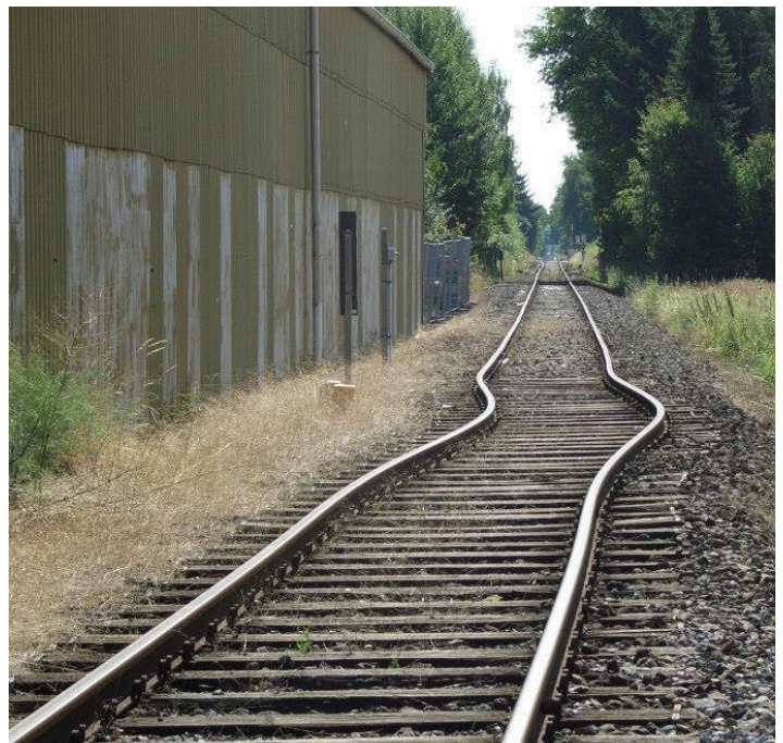
Buckling rails as a result of continuous exposure to heat make train traffic impossible. Credit: Wikimedia
