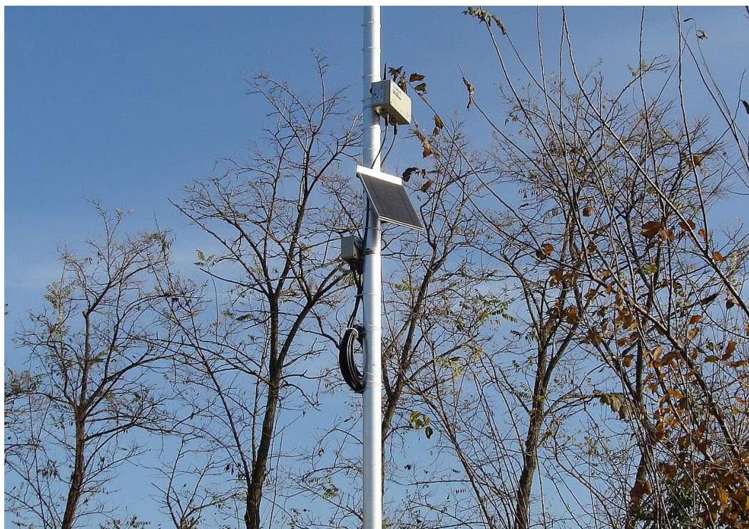
Figure 3. Closer view of the A753 RTU, solar panel and pressure relief box (from up to down)
