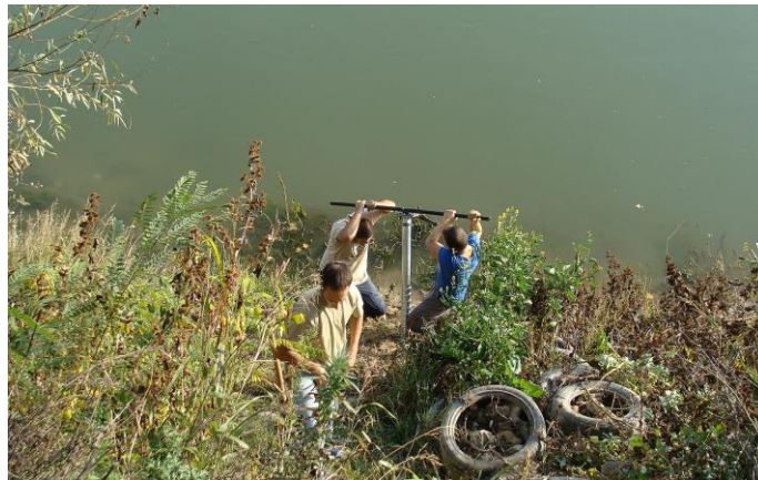
Figure 6. Re-adjustable foundation screws were utilised at locations where the Danube is known as strongly either erode or sediment its banks
