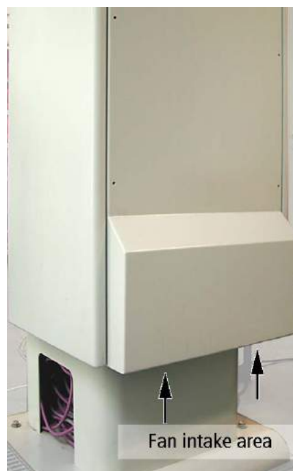
Fig. 29: Fans inlet. Remove snow, sedimentation,...
