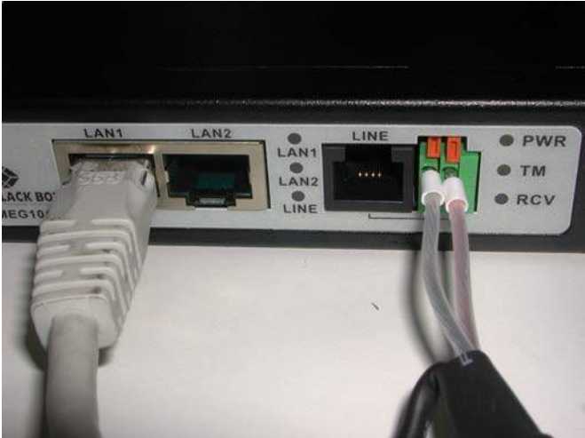
Fig. 11: DSL connection using the Black Box DSL Interface
