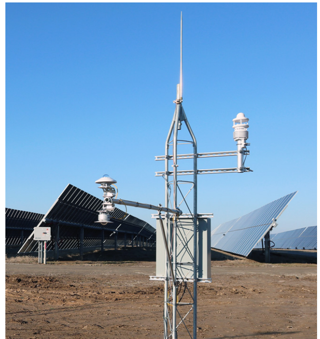
Image displayed is an OTT HydroMet Solar MET Station with Lufft weather sensors and Kipp & Zonen pyranometers.
