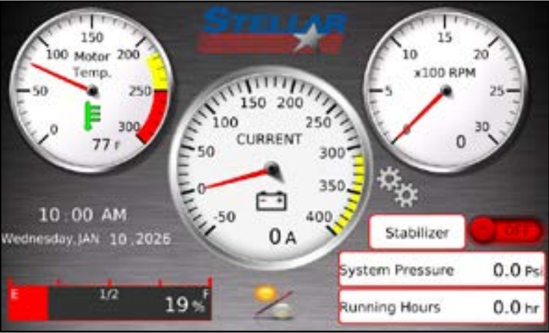
Figure 29: Status of Charge, Low Charge
